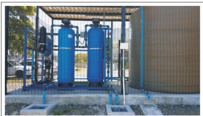
SIDE VIEW OF INSTALLATION.
